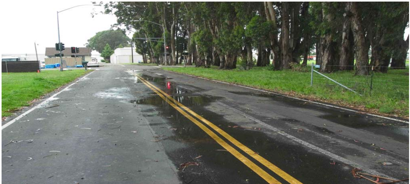
Figure 8.12 PATH Testbed with Standing Water
